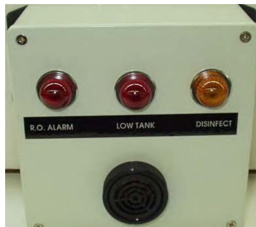
Typical RO Remote Alarm Monitoring Box
