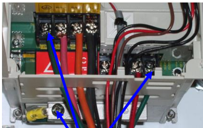
Old Model VFD Three ground wires
