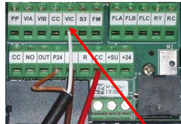
New Model VFD Wire located on terminal post VIC
