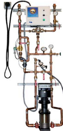
Pre-Treatment Wall Mount Header
